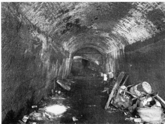
The 'Corner tunnel' in 1998 before restoration. The entrance is located at the back of the Lord Mayor's Stables Yard Photo by Nick Catford
